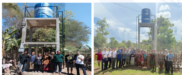
Figure 4: Groundwater Completed Construction System
