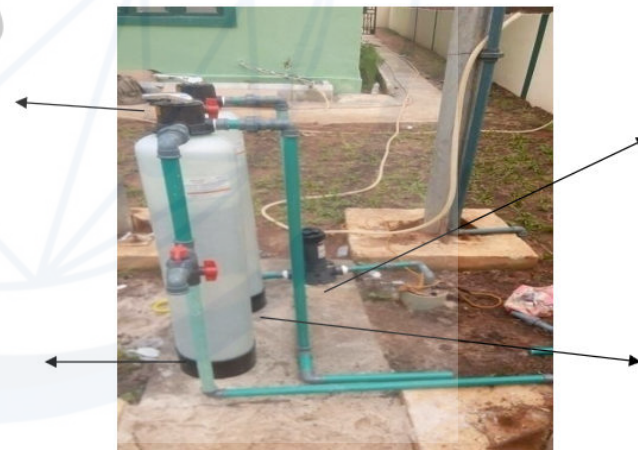
Figures 6: Treatment System Installed for House Use
